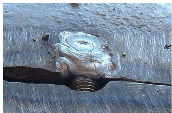
Fig no. 4: Crack
