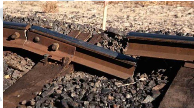
Fig.4: Broken Railway Track
