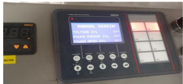
Fig 4: 128*64 Display PLC Module
