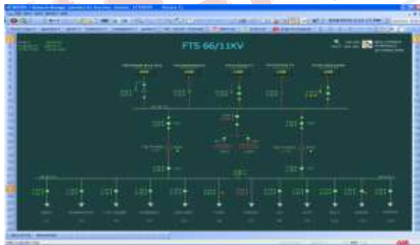
Fig 4. Operator at ALDC can observe single line diagram of 66/11kV substation at control centre
