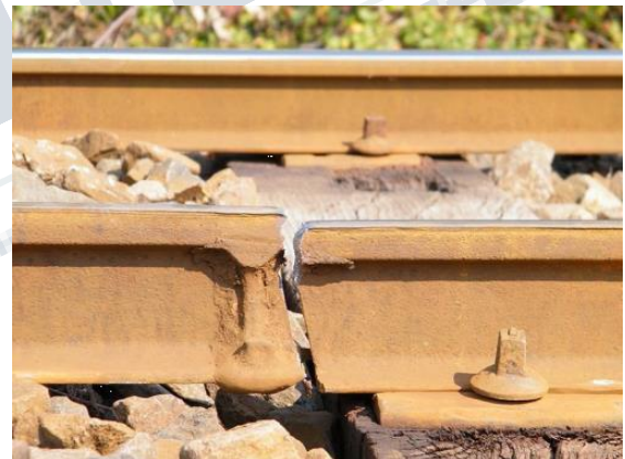
Fig 1: Crack in Railway Track
