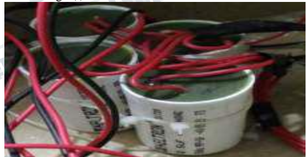
fig.d. Capacitor bank
