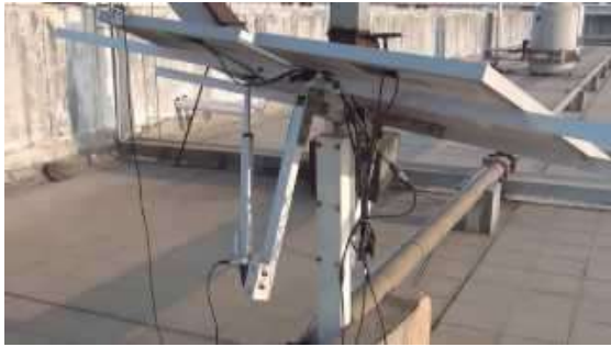
installed prototype dual axis solar tracker
