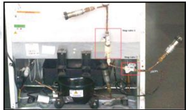
Fig. 2 Stop valve connections at compressor discharge
