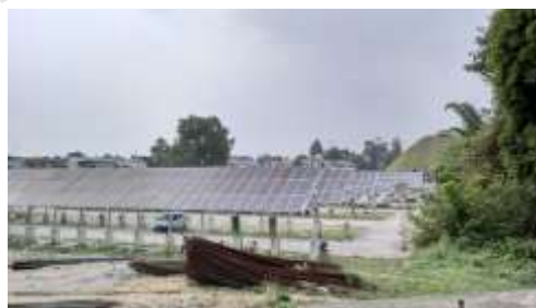
Fig 4. Solar panels on the parking lots
