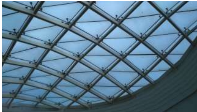
Fig 3. Skylight Covering of the Green Building
