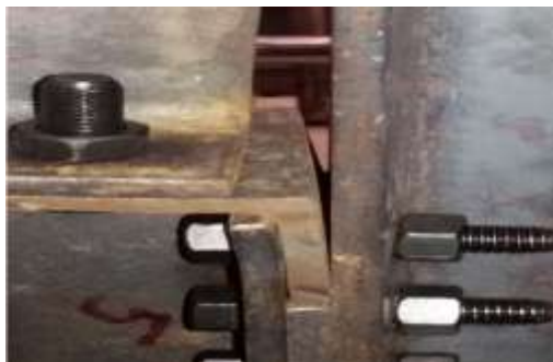
Fig.4. Failure of stiffened seated connection
