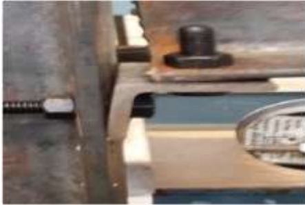
Fig.3. Failure of unstiffened seated connection
