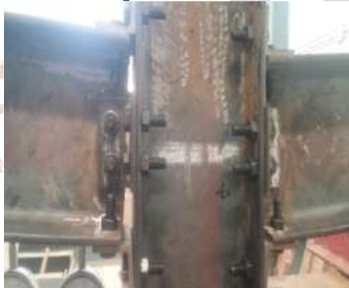
Fig.5. Failure of moment resisting connection
