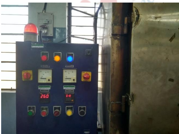
Figure 3. Stress relieving furnace with control panel
