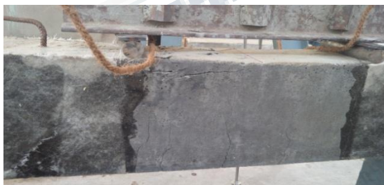
Ultimate failure of strengthened beam 3
