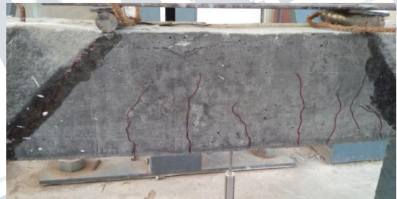
Ultimate failure of strengthened beam 4
