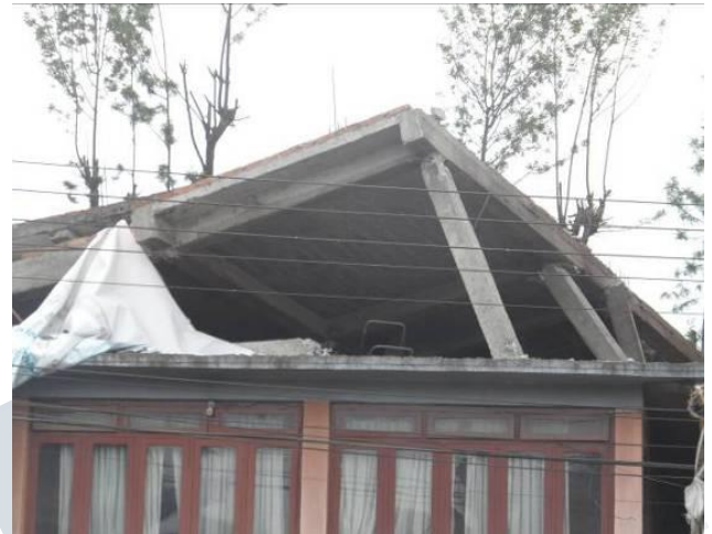
Fig. 11. RC frame 2nd floor collapsed at Jagati, Bhaktapur.
