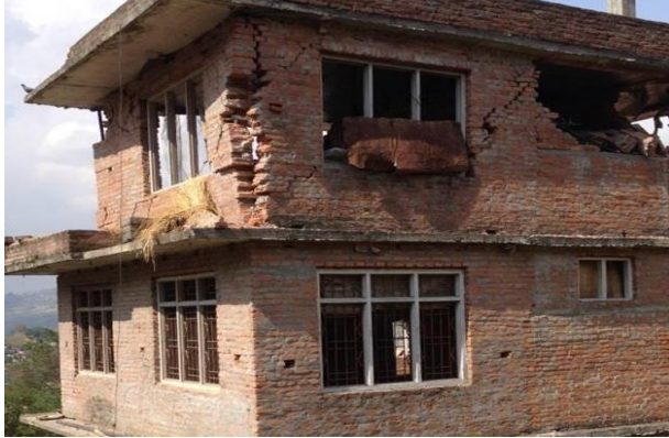
Fig. 10. Damaged Brick in Cement building.
