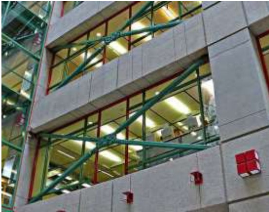
Fig. Concordia's Library Building Connected with Pall Friction Damper
