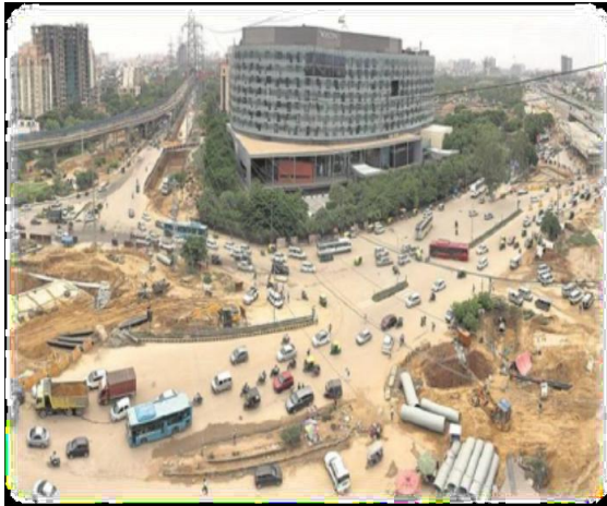
Figure 1 : Encroachment in the Flyover Construction area
