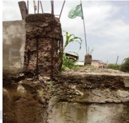
Fig. 7 “Open reinforcement” Source: author
