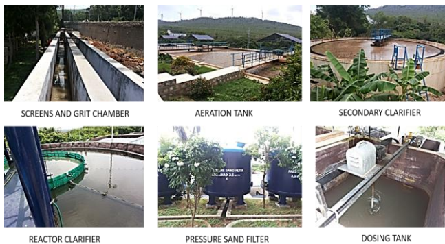
Fig 1 Treatment units in Sewage Treatment Plant, Block-c, Tirumala
