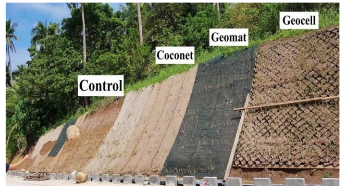
Fig. 2 Illustration of the Field Application of the Geotextiles on Project Site with Vegetation
