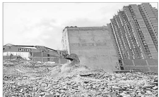
Fig 9: Greater Noida Collapse [13]
