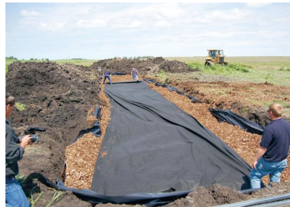
Figure 4. Covering the woodchips with ageo-textile fabric before laying the soil cover at a bioreactor installation (courtesy of the Iowa Soybean Association Environmental Programs and Services)
