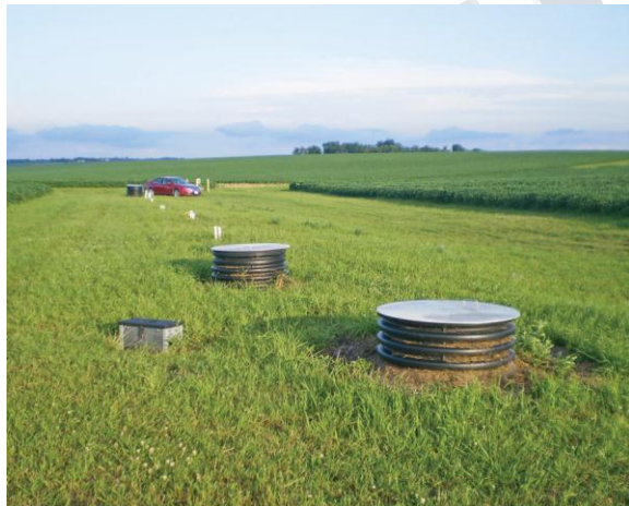
Figure 5. Woodchip bioreactor after installation; circular sumps and PVC wells used for research monitoring (Northeast Iowa Research and Demonstration Farm)
