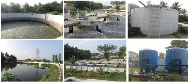
Figure 7 (Clockwise from top left): Collection well; clarifier; settling tank; pressure sand and activated carbon filter; sludge drying bed, and treated water pond with walking track.
