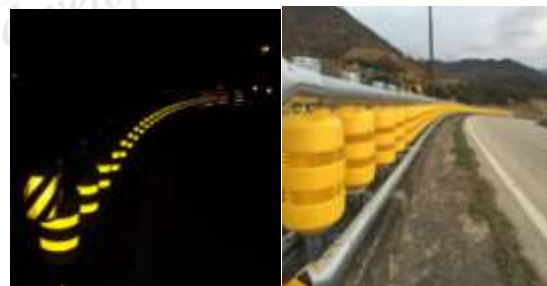
Fig.5 Rolling Barriers during Night and Day Time
