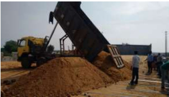
Dumping of Fill Material
